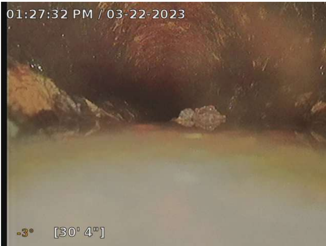
Photo Depicts camera sitting with in stagnant waste water, within eroded bottom area of cast-iron pipe. Also observed within photo is accumulation paper product that had been caught on exposed edge of eroded piping.
